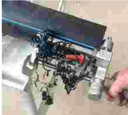
2- Scrape at last 0.2 mm of outside pipe surface to remove oxidation and other contaminants.
